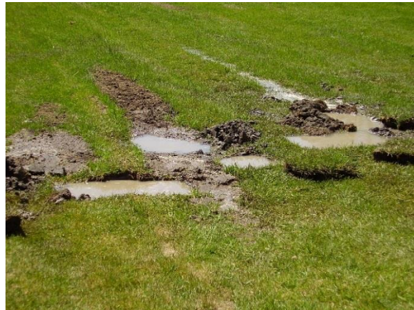
Figure 9: Turf disruption resulting from irrigation pipe failure
