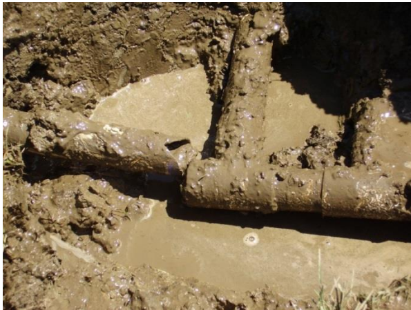
Figure 8: Sport field irrigation pipe failure
