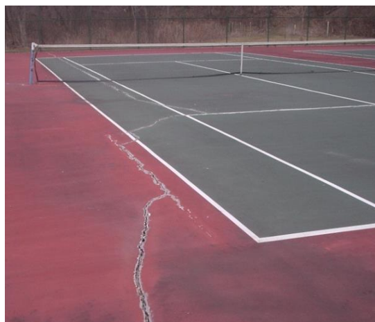
Figure 6: Cracked tennis court surface
